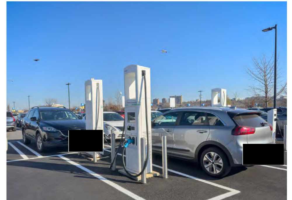
Figure 15. Electric Vehicle Charging
